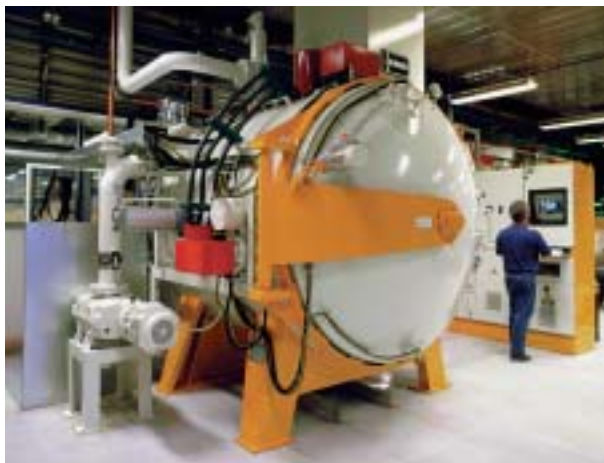
One of the vacuum treatment chambers.
